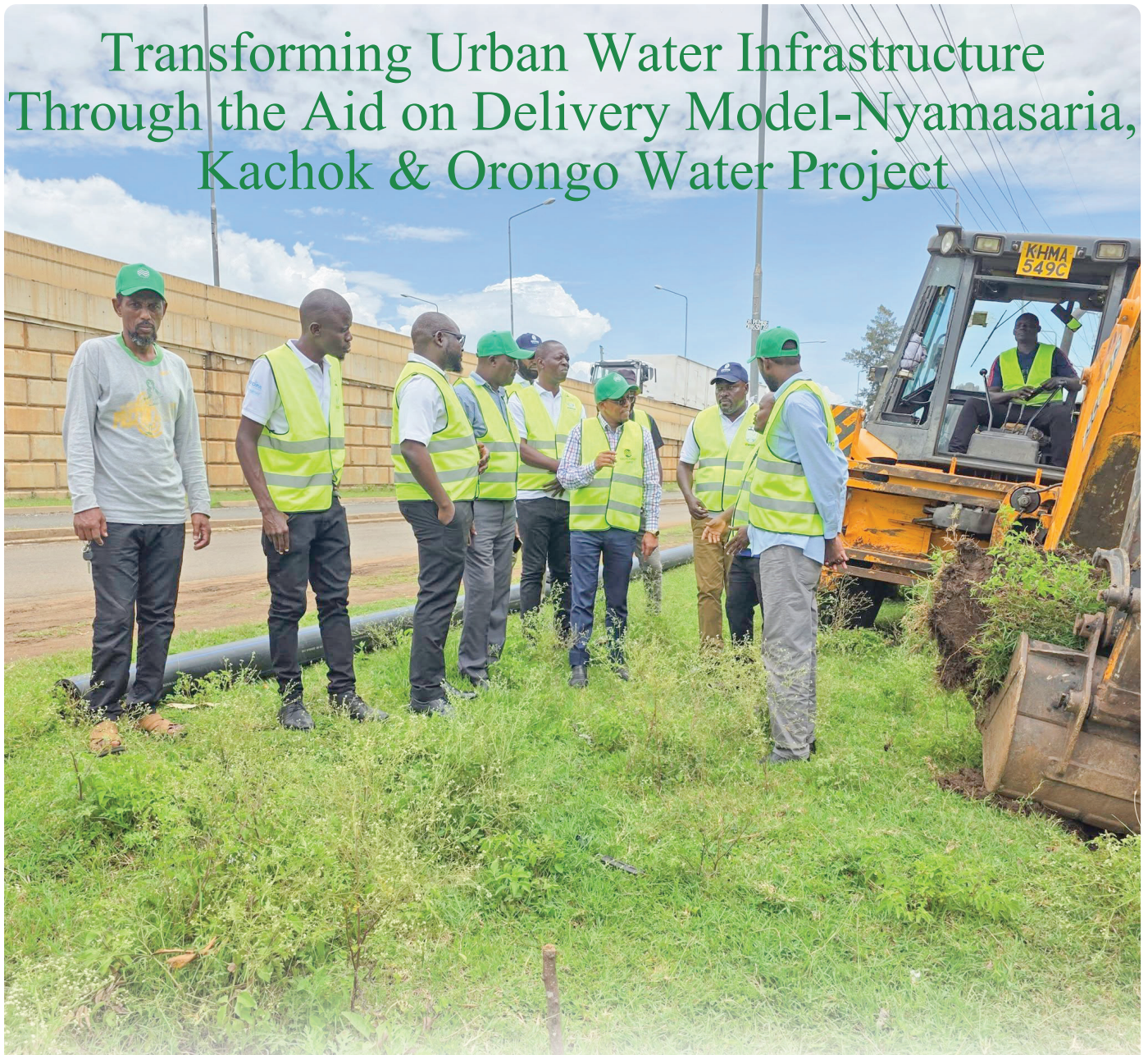
Photo file: Team converge for a debrief with contractor after the ground breaking activity.
